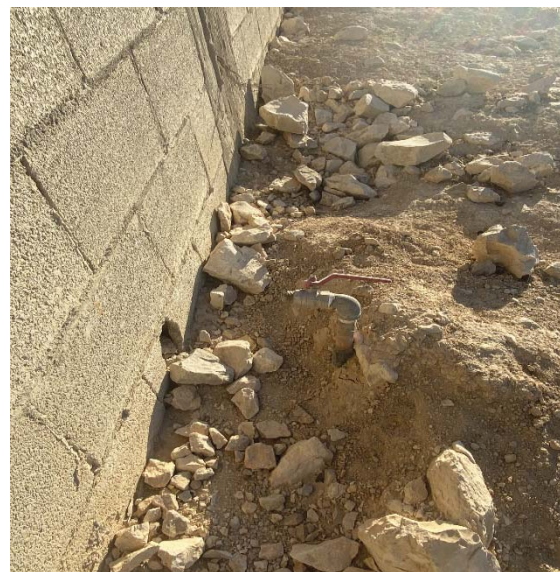
Figure 1 A water pipe and water network installed for Fasayil Al-Fauqa by MA'AN Development Center and the Palestinian Water Authority, but the pipe remains disconnected
