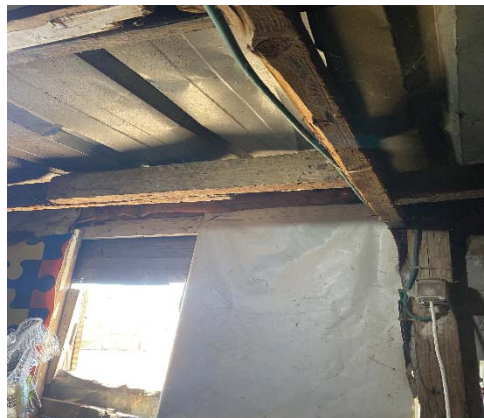
Figure 2 A standard kitchen in the Jaba' community exhibiting substandard and hazardous construction.
